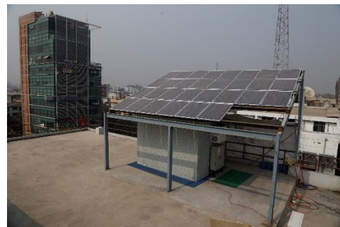
Fig: Solar PV- Diesel Hybrid Mini Cold Storage on the rooftop of UIU University
