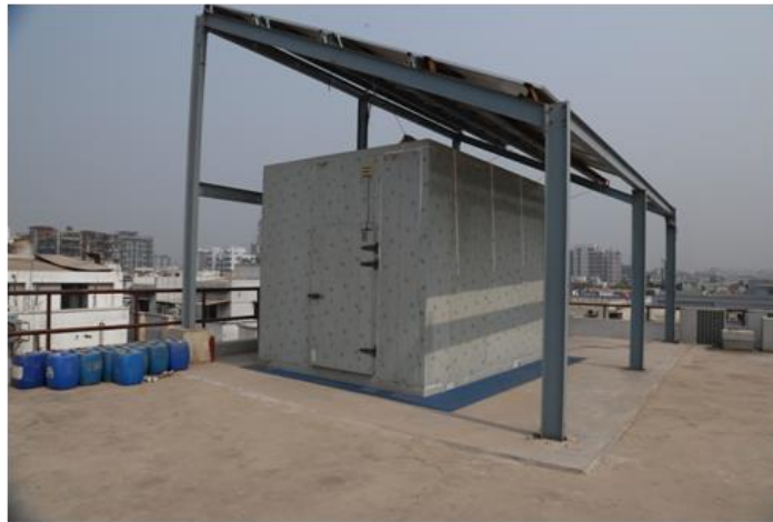
Picture of the of the actual Cold storage fabricated at the roof top of United International University
