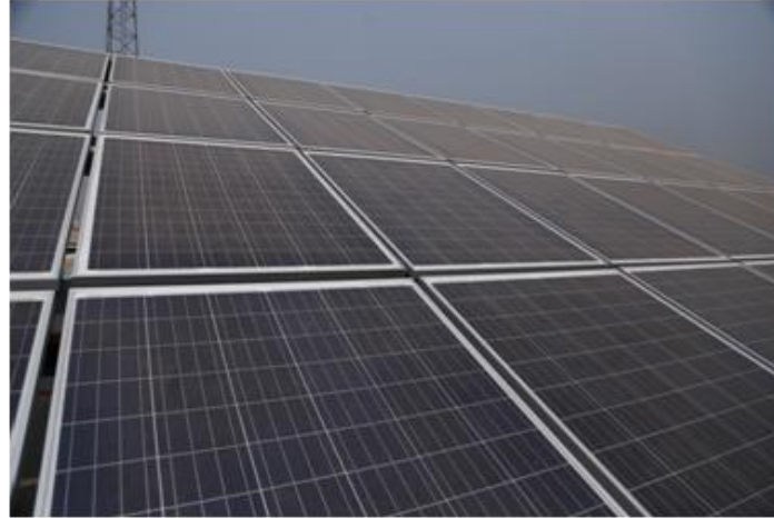
Picture of the solar panels used in the cold storage
