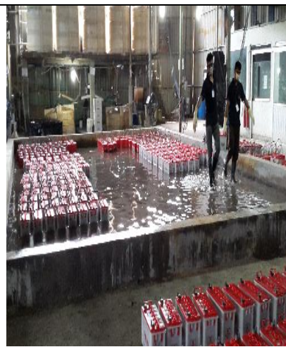
Photograph : A view of charging unit
