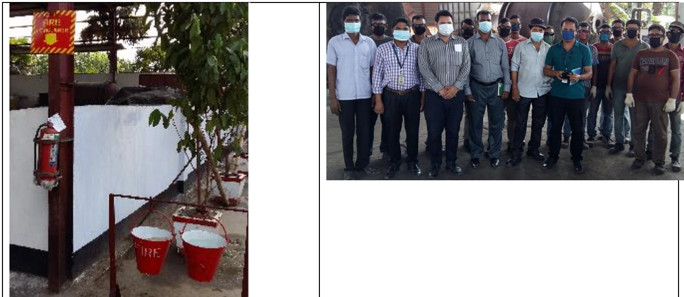
Photograph : Firefighting arrangement
