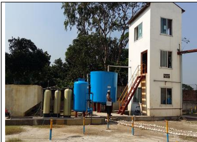
Photograph : View of 120 m 3 /day ETP
