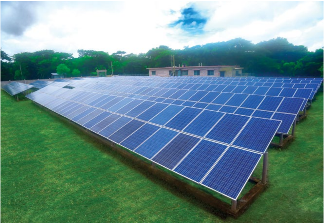
Solar mini-grid project financed by IDCOL
