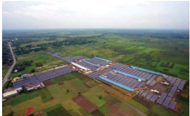
8 MW Utility Scale Project by Sympa Solar Power Ltd.
