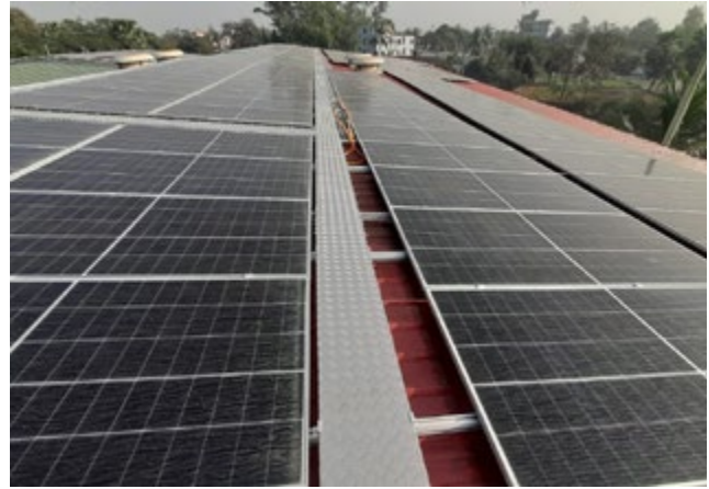
2.67 MWp rooftop solar project on the rooftops of Hatil Complex Ltd.
