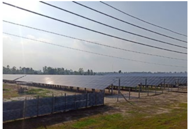
2.87 MWp rooftop solar project on the rooftops of Kazi Farms Ltd.
