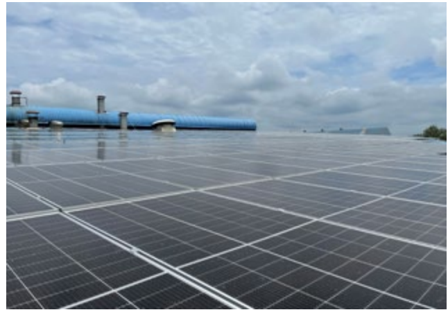
3.23 MWp rooftop solar project on the rooftops of Comptex Bangladesh Ltd. by Joules Power Ltd. (JPL).
