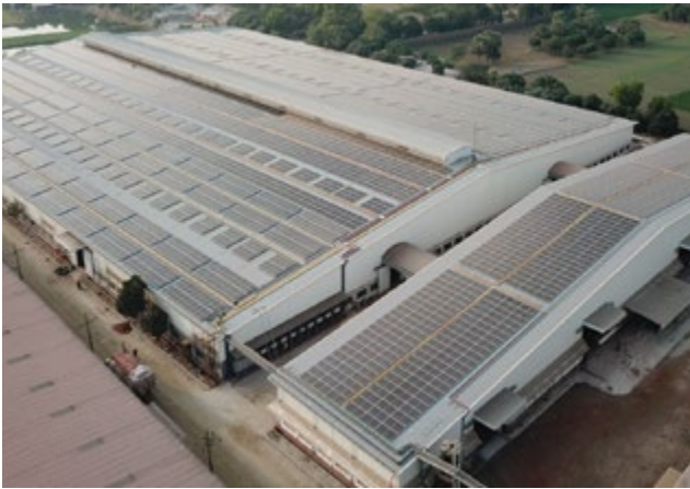
2.4 MWp rooftop solar project on the rooftops of Janata Jute Mills Ltd.
