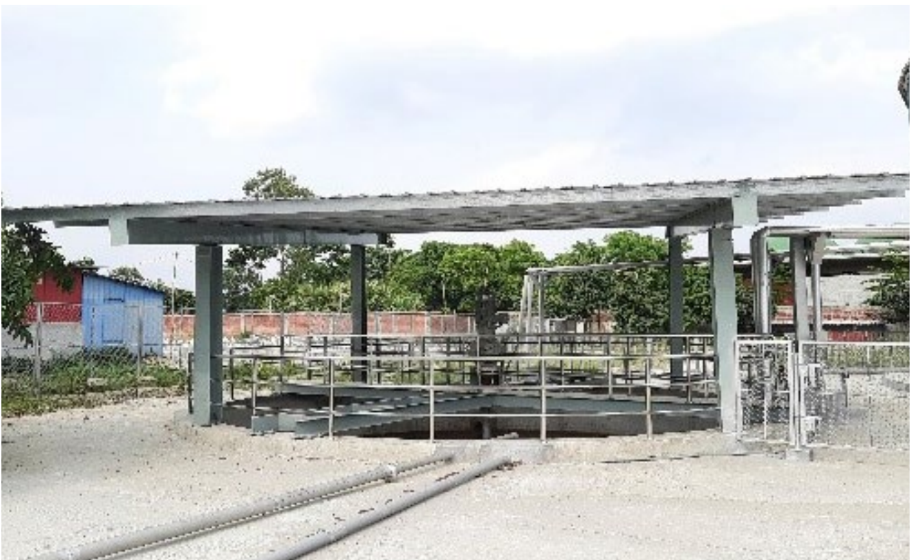
400 kW Biogas based Electricity Project at Satghoria, Halodia, Louhajung, Munshiganj
