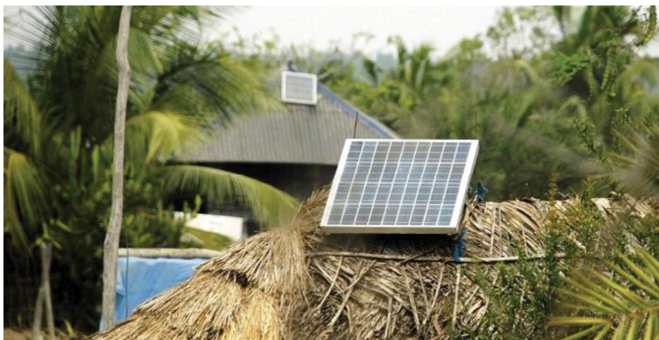
Solar Home System providing electricity in rural off-grid areas.
