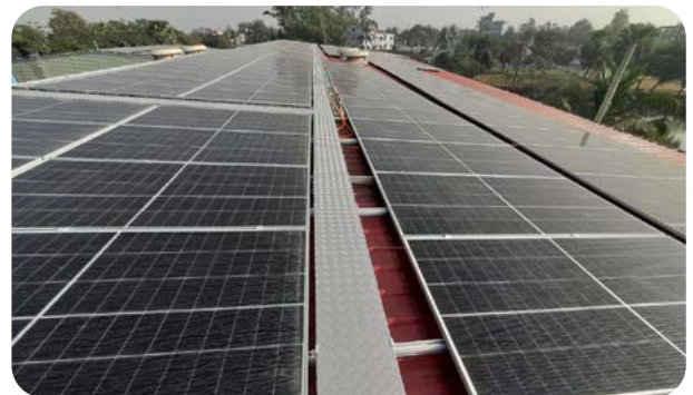
2.67 MWp rooftop solar project of Hatil Complex Ltd.
