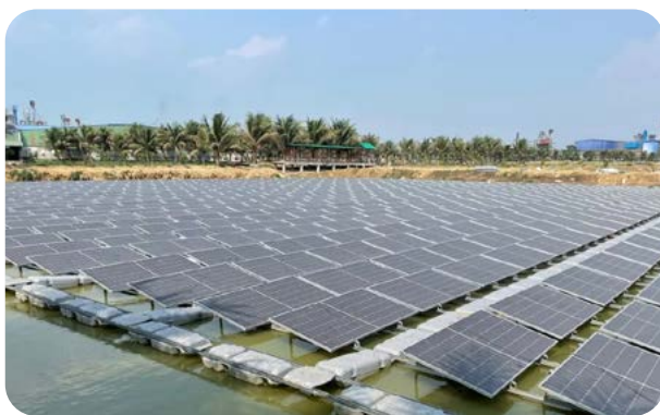
784 kWp solar PV system of Nawab Auto Rice and Feed Mills located at Chapai Nawabganj
