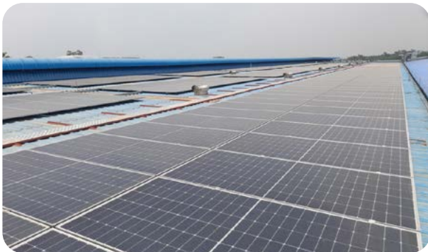
991.44 kWp rooftop solar project of RANCON Infra. and Engineering Ltd.
