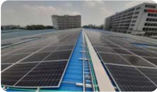
5.00 MWp rooftop solar project of Transcom Beverage Ltd.
