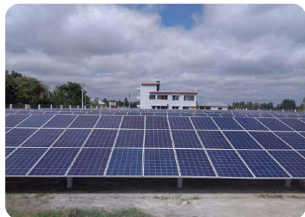
250 kWp Solar Mini-grid project implemented by Solar Electro BD
