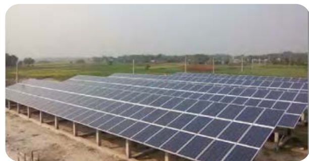
228 kWp Solar Mini-grid project implemented by Super Star Group
