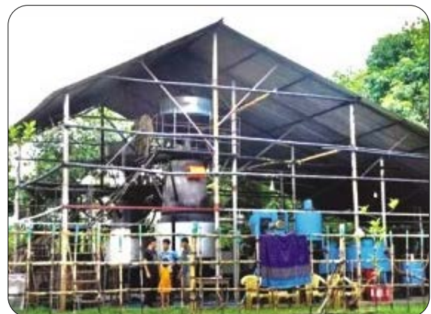
400-kWp rice husk gasification-based power plant of SEAL
