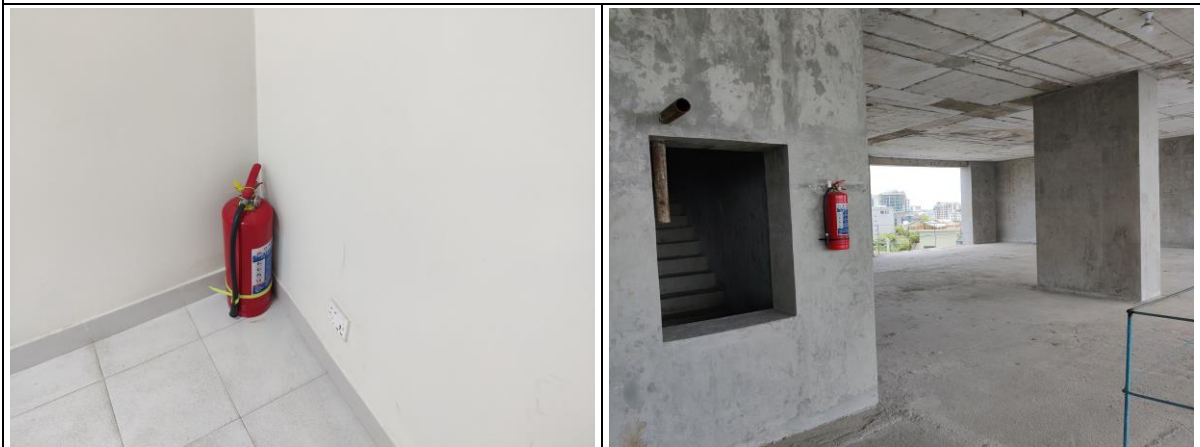
Photographs of firefighting equipment, fire safety materials
